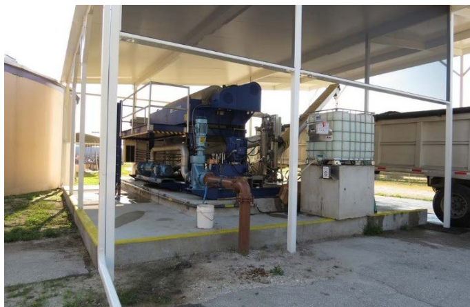
Figure 2: Sludge Dewatering Facility
