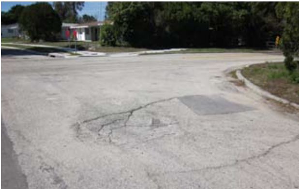
Roadway Subsidence along Storm Sewer near Shade Avenue
