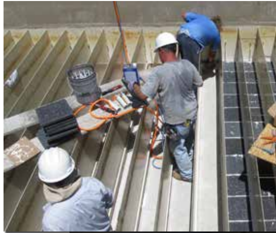
Aluminum oxide plates being installed by TLC Diversified, Inc. of Palmetto, FL, during the 2012 filter rehabilitation at the Manatee Southwest WRF.
