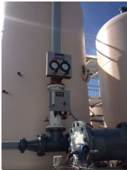
Anion Vessel Influent In-Line Aerator
