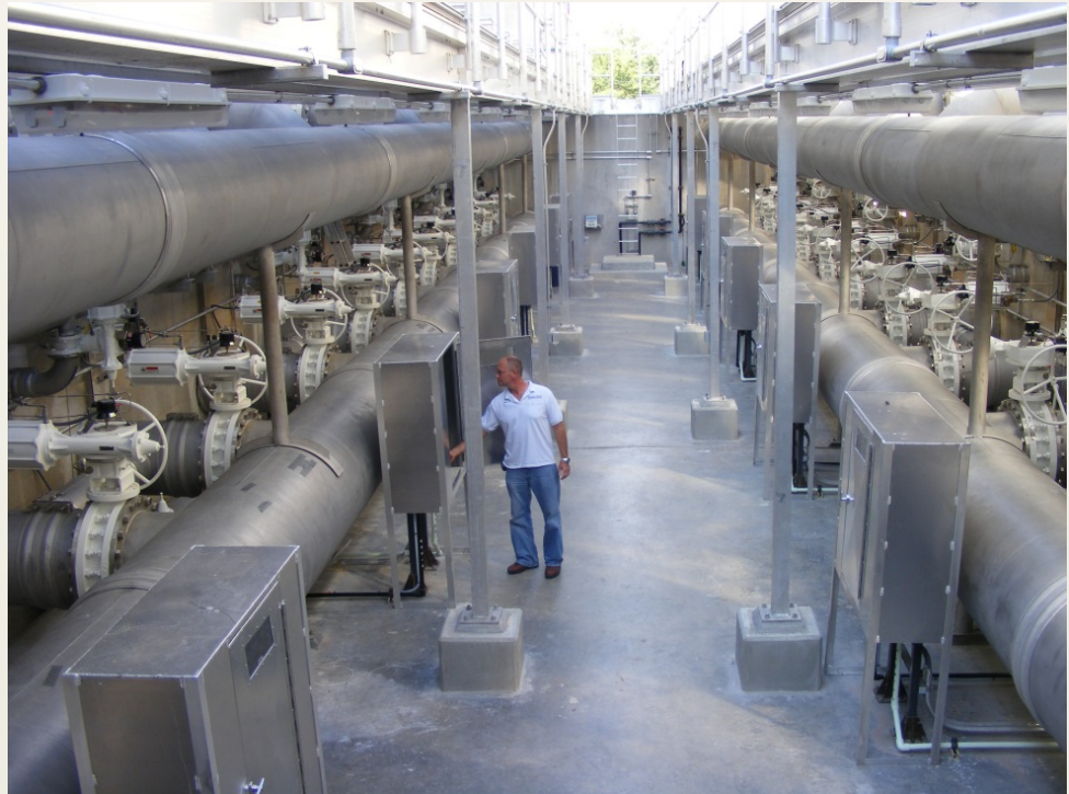
Mike Chell, Operations Supervisor, Checking Filter Effluent Turbidimeters
